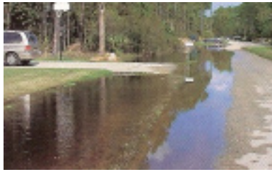
Awaiting swale repair
