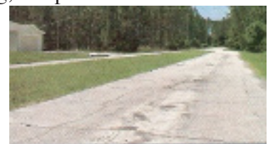
Awaiting road repair
